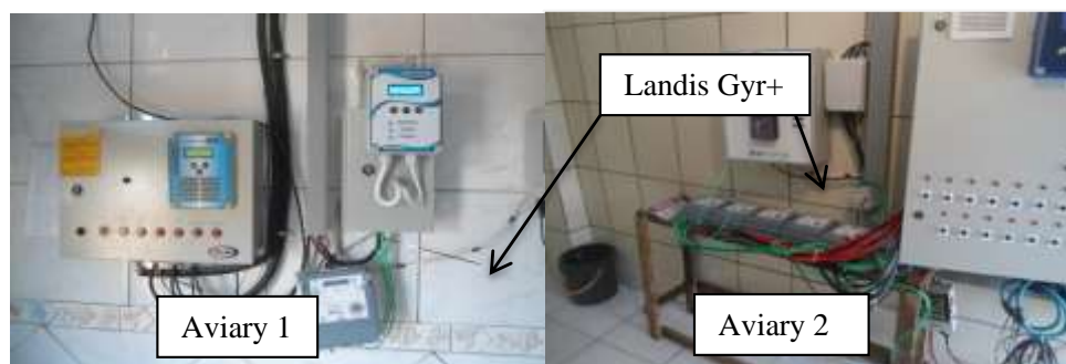
Figure 4. Measuring instruments installed in the scenarios 1 and 2.
