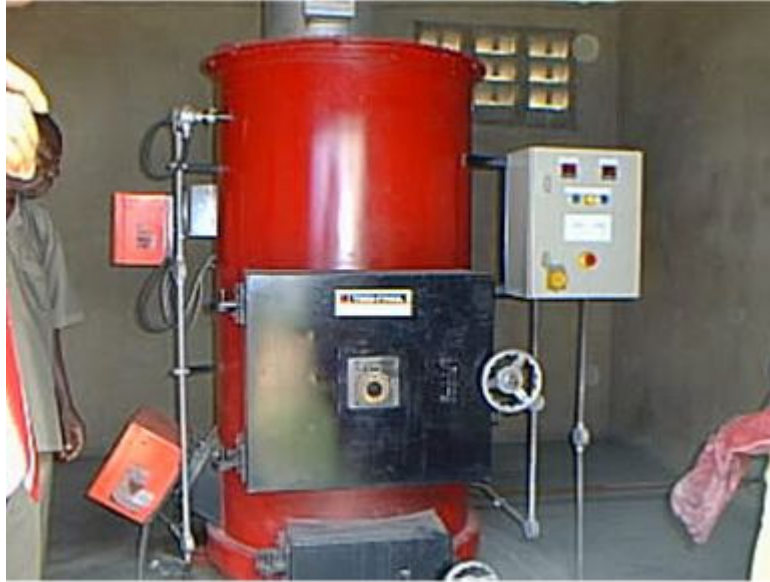
Plate 4. Over-utilized incinerator at UCH Ibadan.
