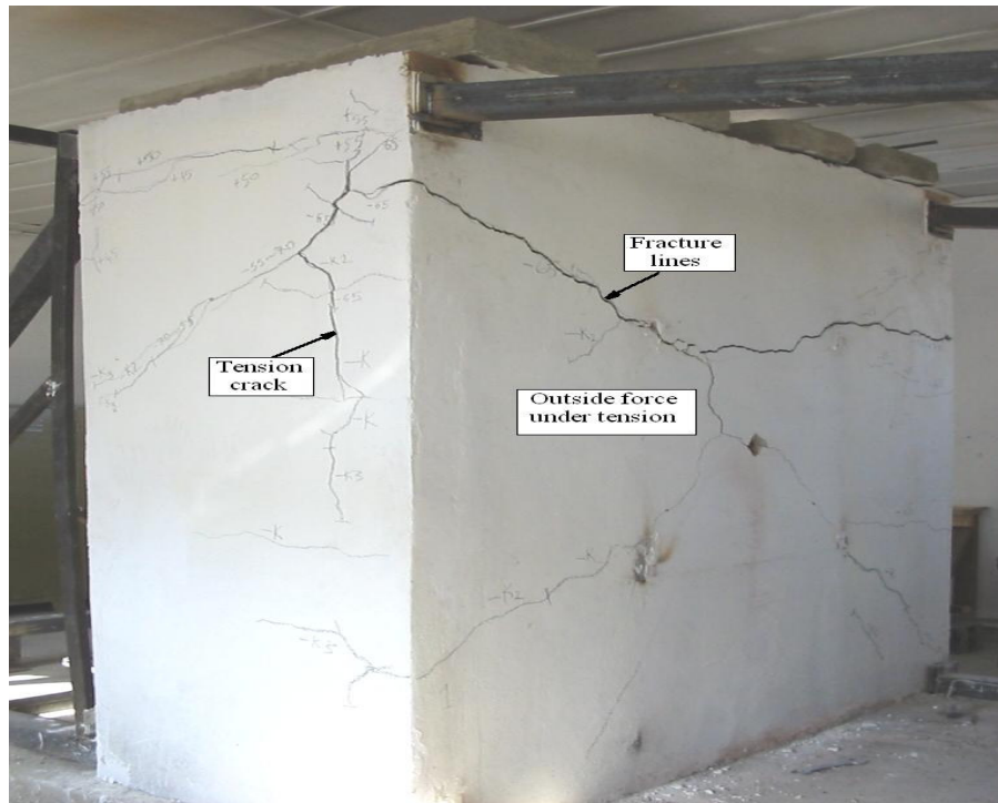
Figure 13. Crack formation at outside surface of URM test wall at final failure.
