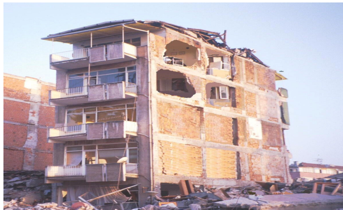
Figure 5. Out-of-plane failure of an URM wall in a low-rise multi-storey building.
