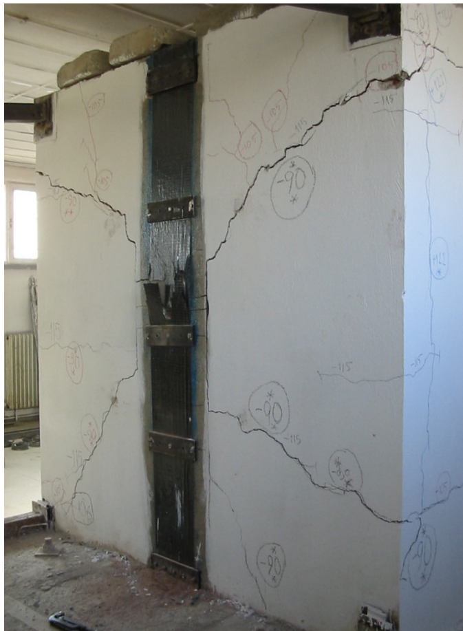
Figure 21. Final failure of the strengthened URM wall S_{(FRP)} by rupture of the FRP strip.
