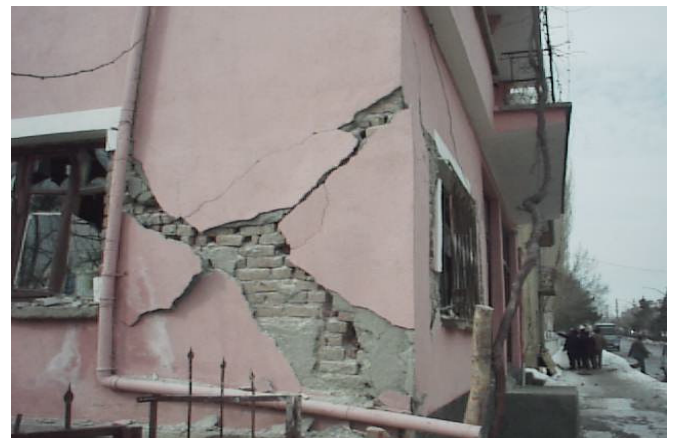
Figure 4. In-plane shear failure of the URM wall.
