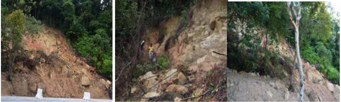
Figure 2. Landslide at 3.9 km Tun Sardon road of Penang.
