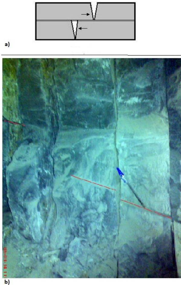
Figure 8. Sliding of (a) step-over fracture, and (b) step-over fracture in wall of tunnel.
