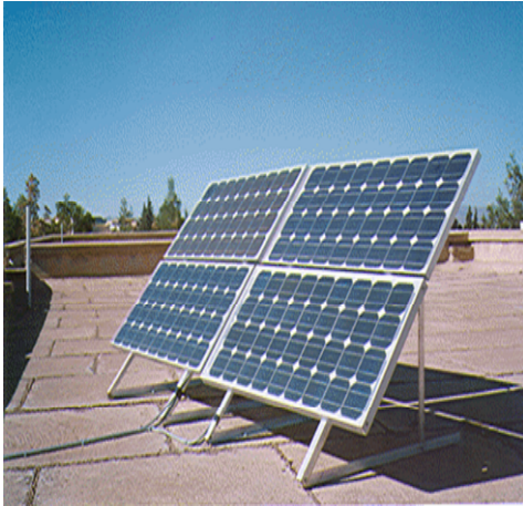
Figure 12. Photovoltaic panels SP75 installed in laboratory.
