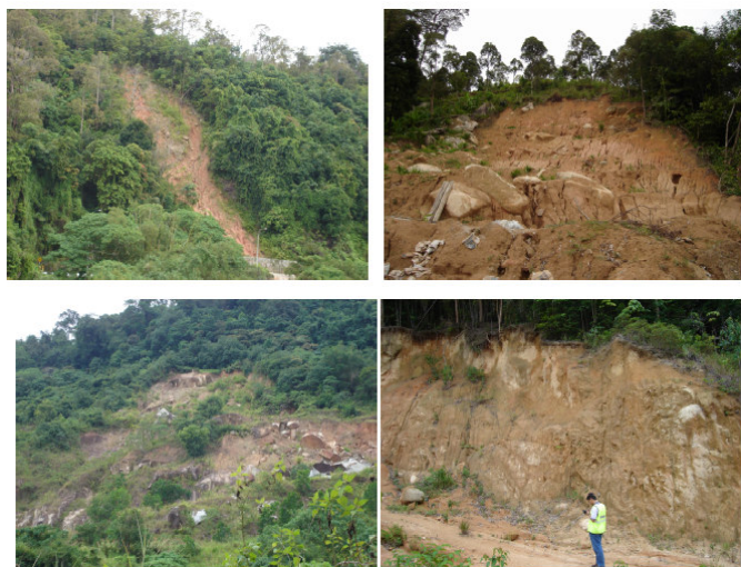
Figure 2. Field photographs illustrating the characteristic and types of landslides in Penang Island.
