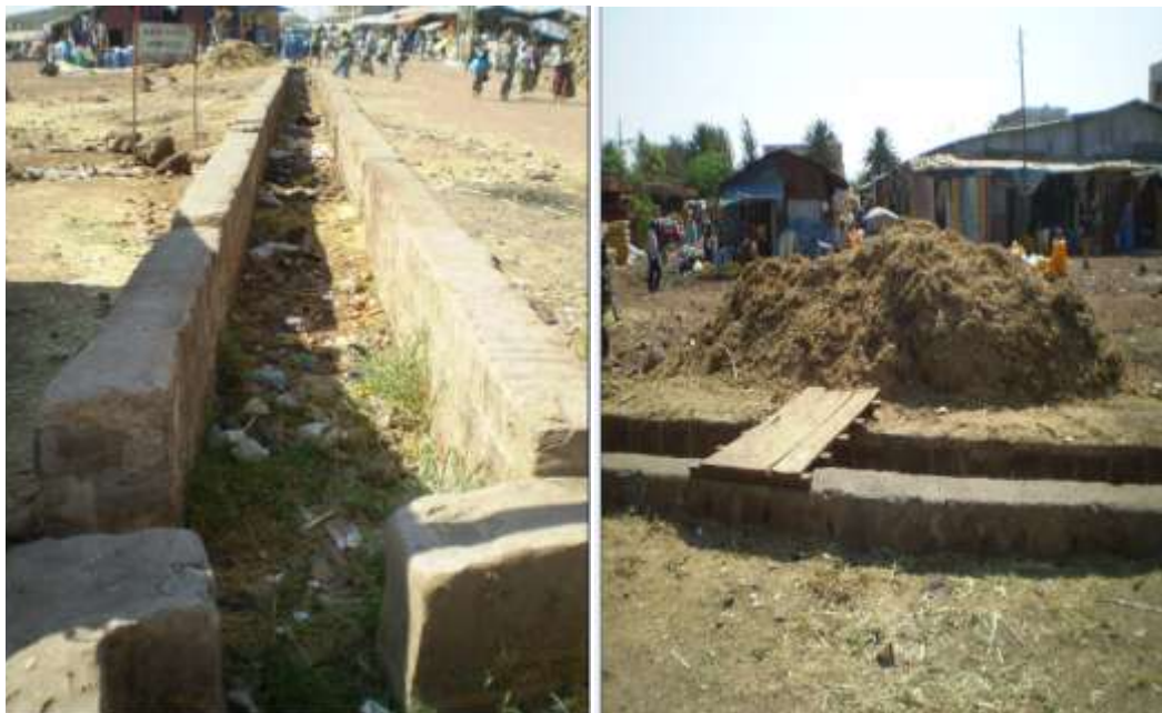
Figure 2. Dumped waste at open place and channel.
